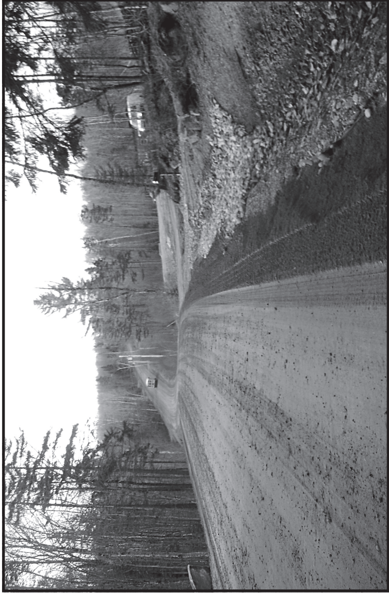
Spring Flood 2014 Repairs East Hill Road Photo by Eden Highway Dept.
